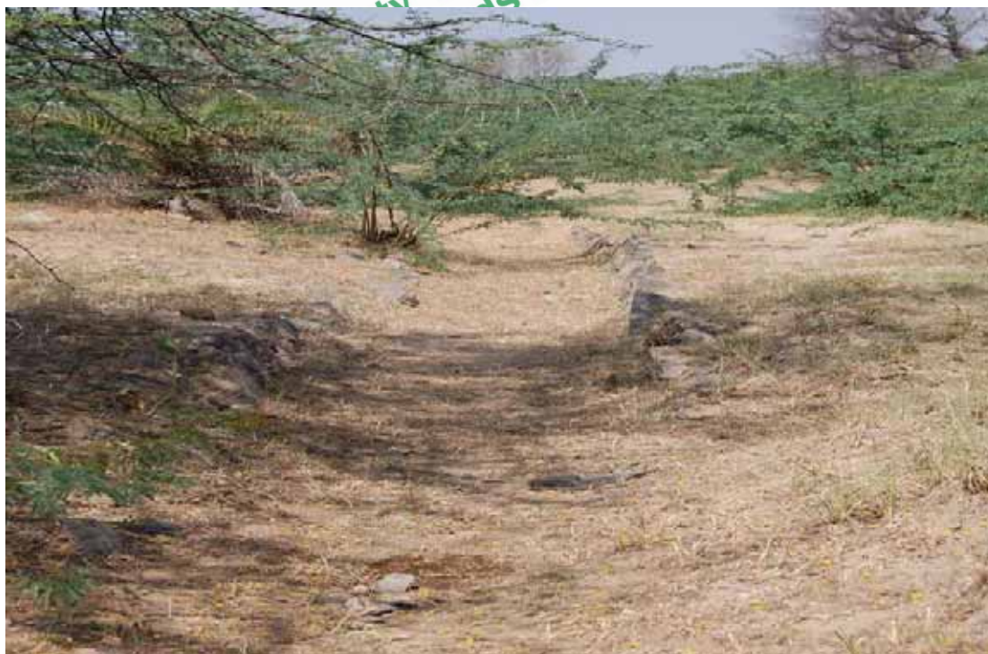
Plate 1 : Drainage line clogged.
